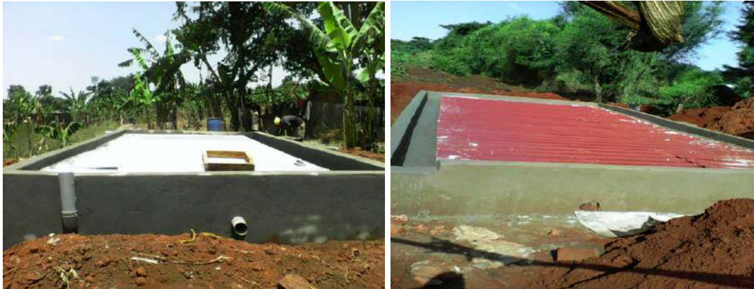
Open surface rain water tanks
