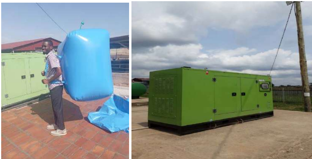
NaLIRRI portable biogas unit (left) and 75 KVA generator operated by biogass (right)
